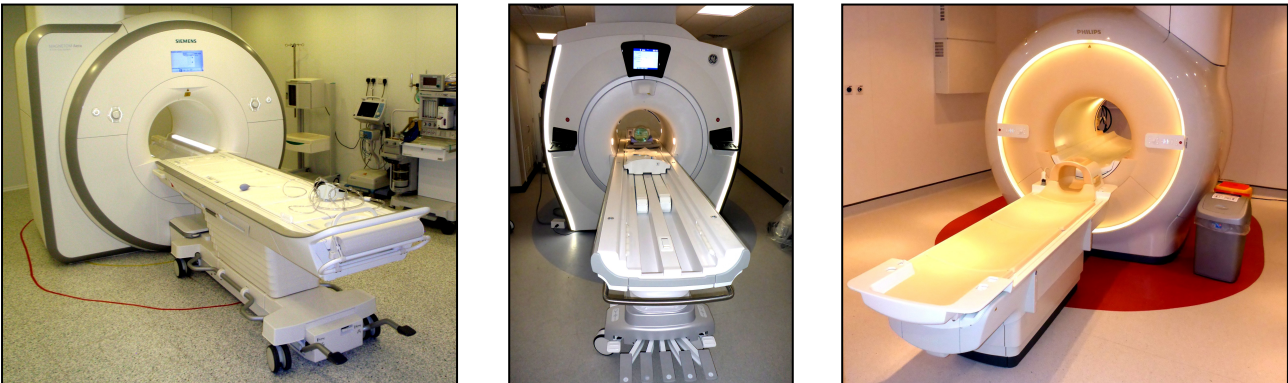
Figure 9: Examples of suitable floor marking within the MRI scanner room to aid safe working practices with regard to MR Conditional ancillary equipment.
